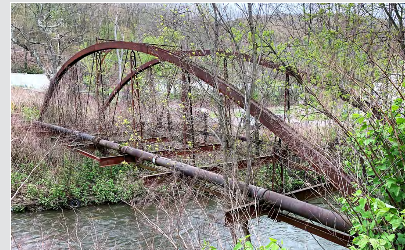
The bowstring in its second location, crossing the Schuylkill River between Mount Carbon Borough and State Route 61. The water line was added to the bridge in 1924.
